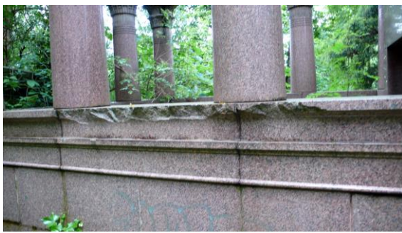
View of damaged section
